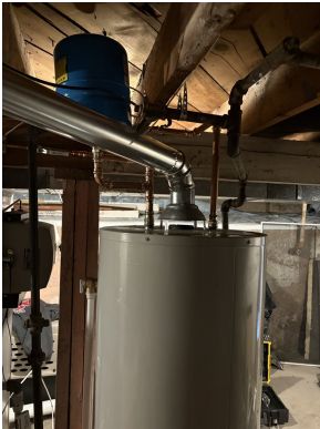
AFTER - rigid flue, supported tank
