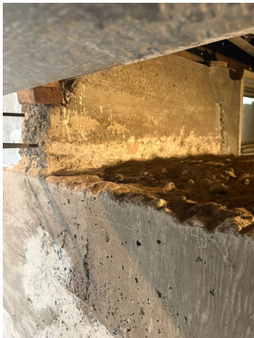
BEFORE - spalled beam pocket
